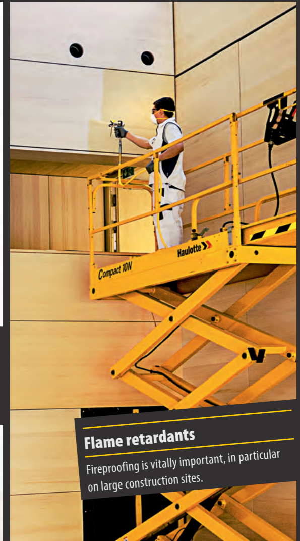
Spraying textured plasters indoors The machine application of fillers saves effort and time. It is the economic, efficient, intelligent way to work on-site.
