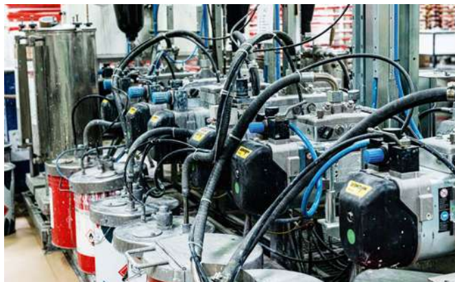
Neelsen uses several high-pressure double diaphragm pumps from Wagner.
